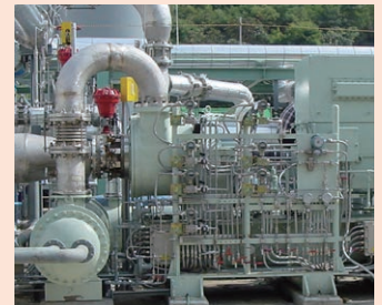
Fuel Gas Compressor
